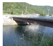
Photo Corrosion of steel plate girder bridge
